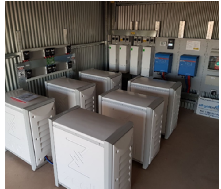
Off-Grid 60kWh battery + 18kWp solar
