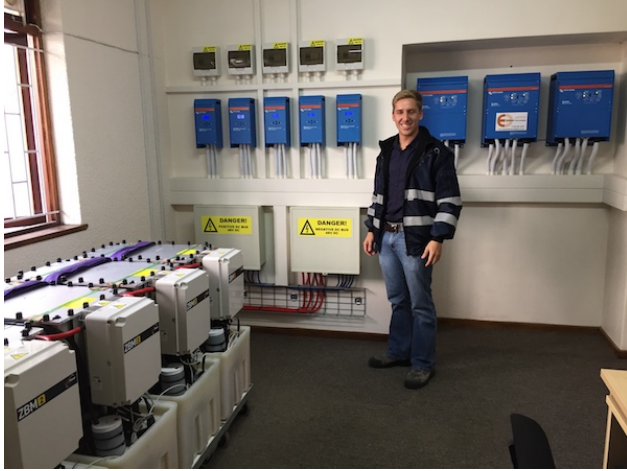
40kWh solar self-consumption system
