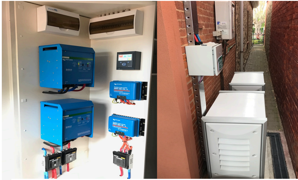
On-Grid 20 kWh / 7kWp solar time-shift + backup
