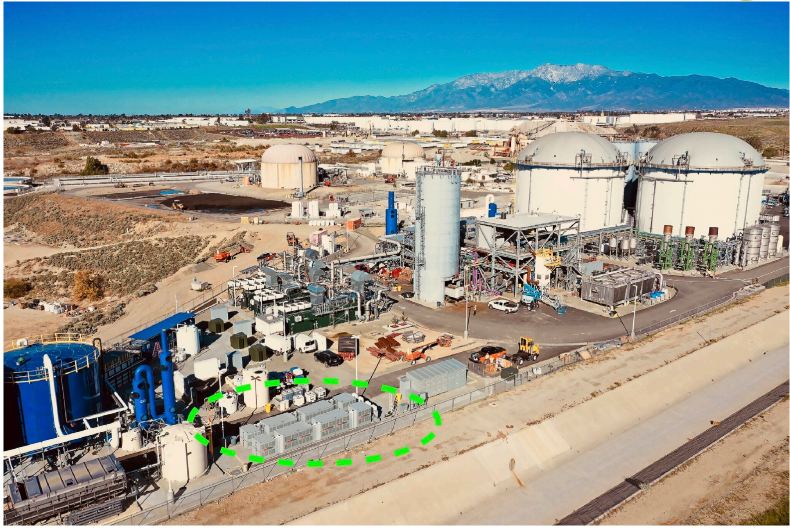
2MWh energy storage system for the Anaergia Rialto Bioenergy Facility in southern California
